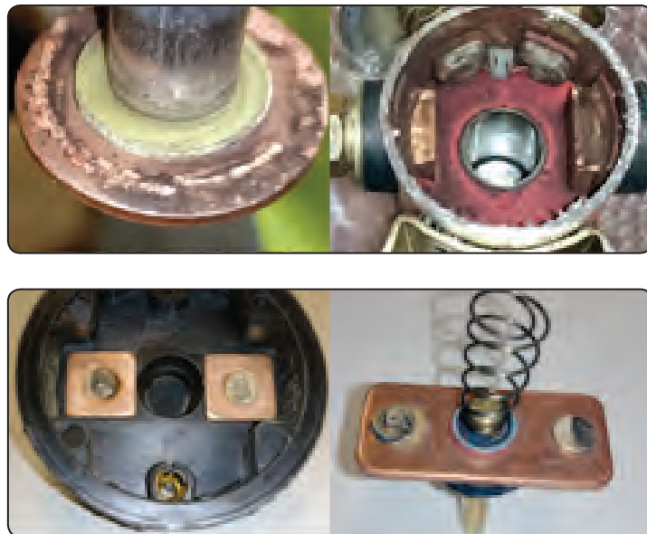
Examples of contactor tips that have momentarily fused together
